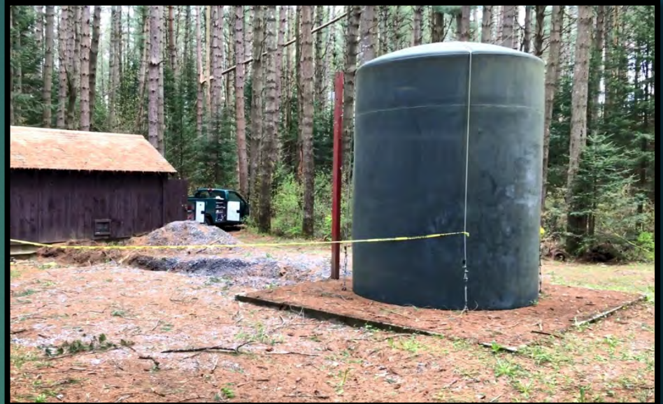
Water Storage Tank
